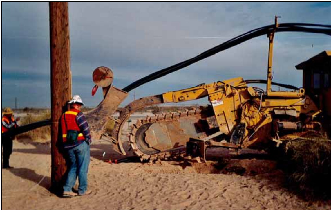
Photo 12. Photo depicts trench rig for installation of multiple conduit lines during Level 3 fiber optic line installation; however, AT&T proposes one conduit line. Cable is installed simultaneously as the trench is dug.
