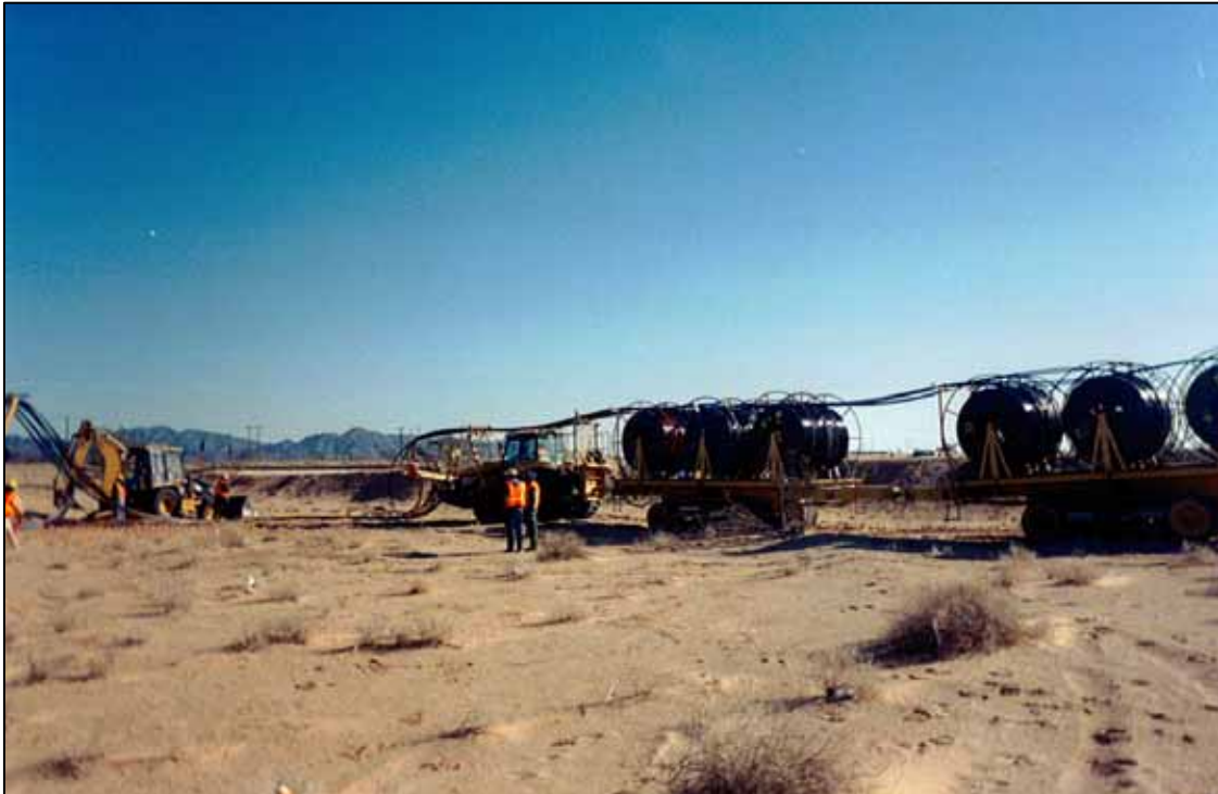
Photo 11. Photo depicts representative construction equipment for installation of multiple conduit lines during Level 3 fiber optic line installation; however, AT&T proposes one conduit line. Note the reels of conduit attached to trench rig.
